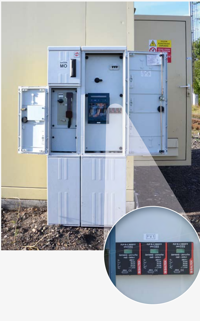
Fig. 2 View to power distribution box of signalling system with installed SPD Type 1 and 2 FLP-B+C MAXI V/3
